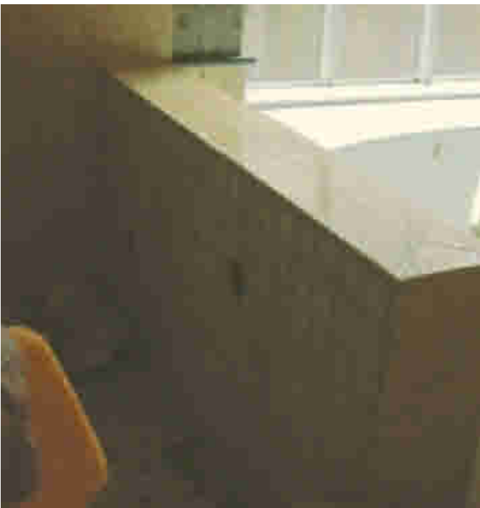
(Below) Showing the pony wall that separates the shower from the tub and where the new glass shower wall will be installed.
