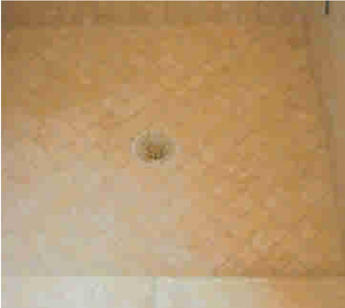
(Above) Completed shower floor set on a diagonal with plenty of slope to draw the water to the center.
