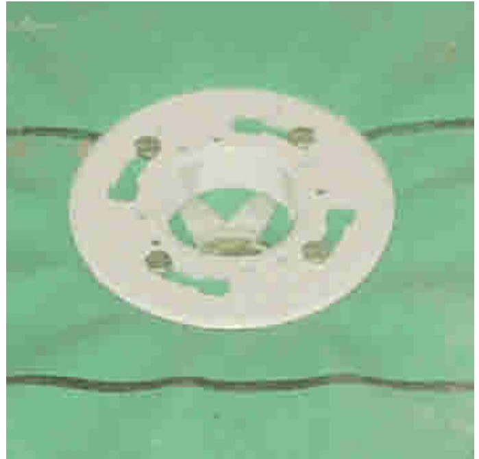
(Above) Close up of the strainer base.
