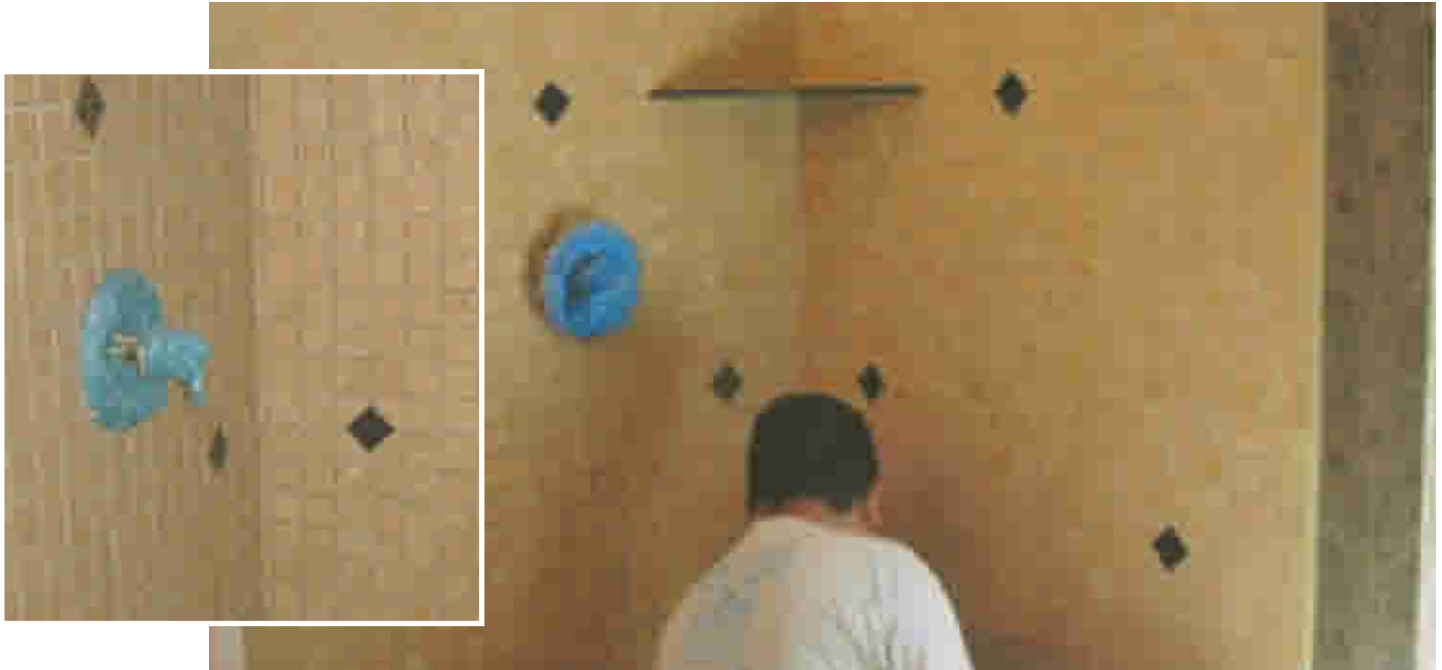
(Above) Granite shampoo ledge being installed, as well as grout being applied to the near finished product.
